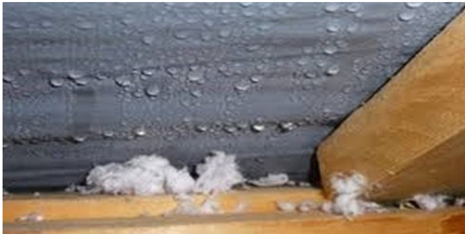
Condensation under the roof
